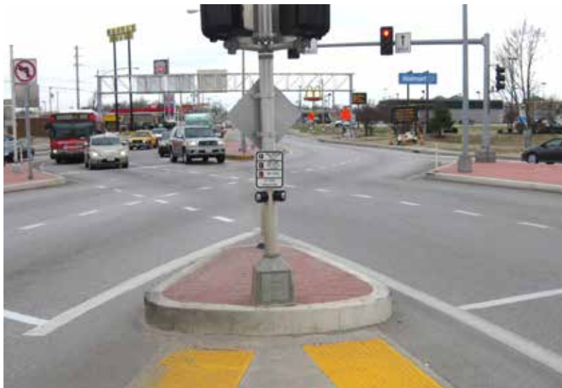
Exhibit 8-10. Undesirable use of single pole with two pedestrian push-buttons, and insufficient separation of the two detectable warning surfaces. (26)
